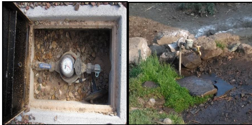
Fig no 3 Water Metering for Private and public connections
