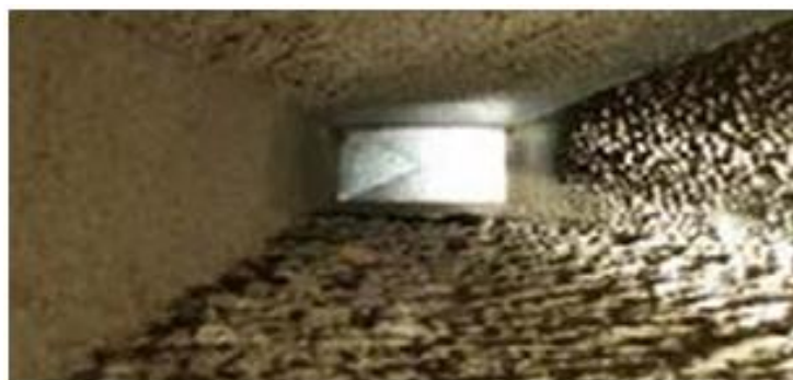
Figure 1 Air duct accumulated with dust
