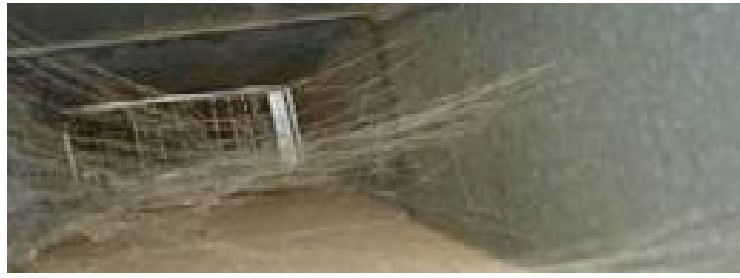
Figure 2 Presence of insects in the air ducts
