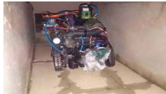
Figure 7. Tread driven movement in air duct
