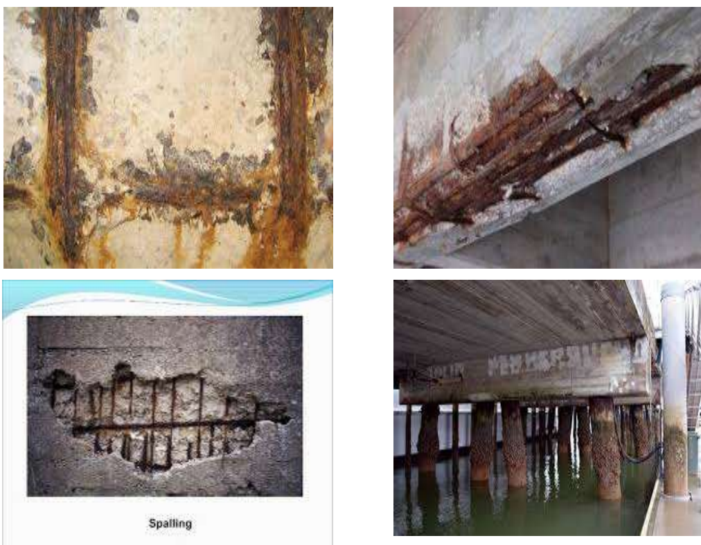
Figure 1: Some images of chloride ion contaminated concrete in coastal region
