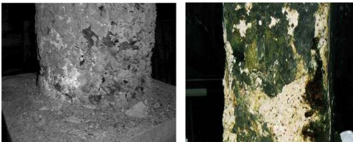
Figure 2: Some images of sulfate ion degraded concrete in coastal region
