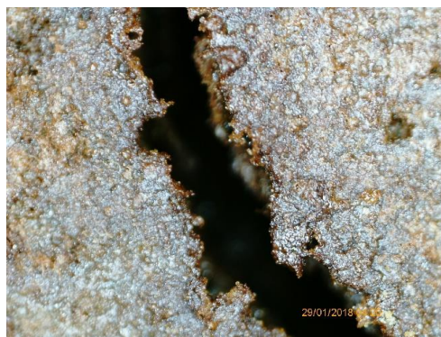
Corrosion level = 235.47 mg/cm 2
