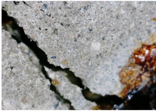
Corrosion level = 93.39 mg/cm 2
