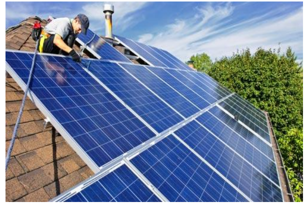
Figure 1: A Solar Array
