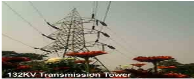
Figure1: -High-voltage transmission lines
